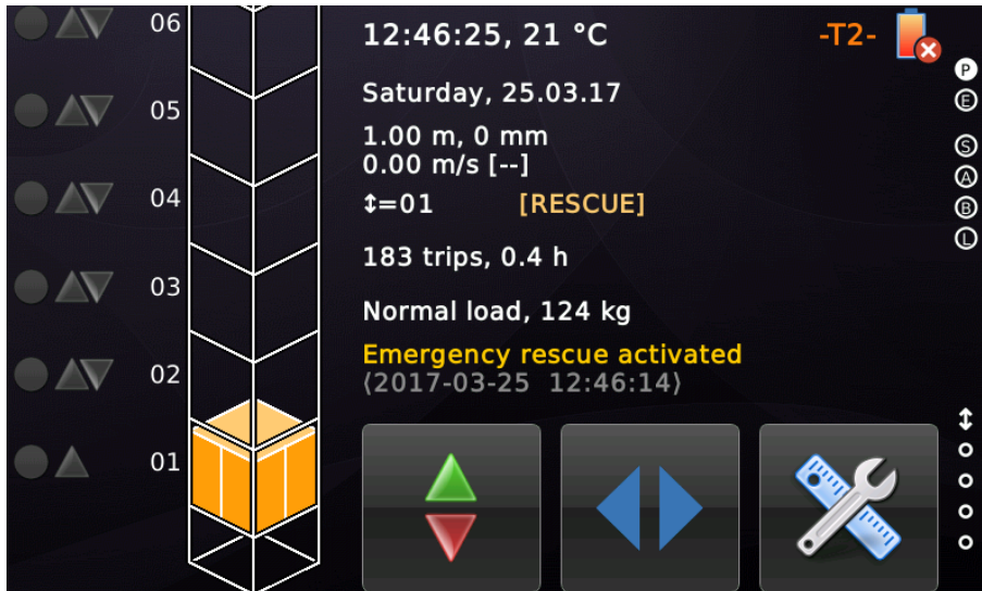
Figure 29: Lift being on inspection/emergency rescue operation.
